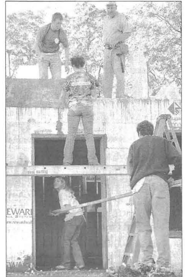
Jenny Heinz, junior, graphic design, ducks beneath makeshift scaffolding at the Habitat site Saturday morning as Mike Rogan (on roof, at left), junior, criminology helps out on the roof. Rogan is with Alpha Phi Omega, a service fraternity which works with Habitat for Humanity on the first Friday of each month.
